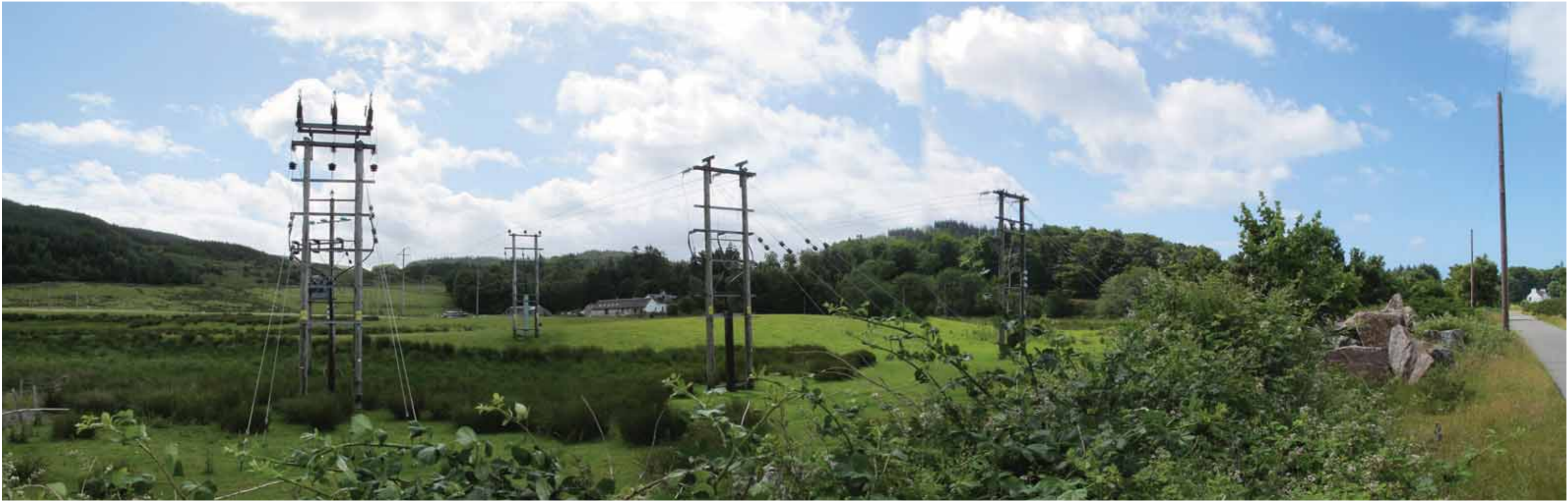
CB38 - Overhead transmission lines and Killlail from the B8000
