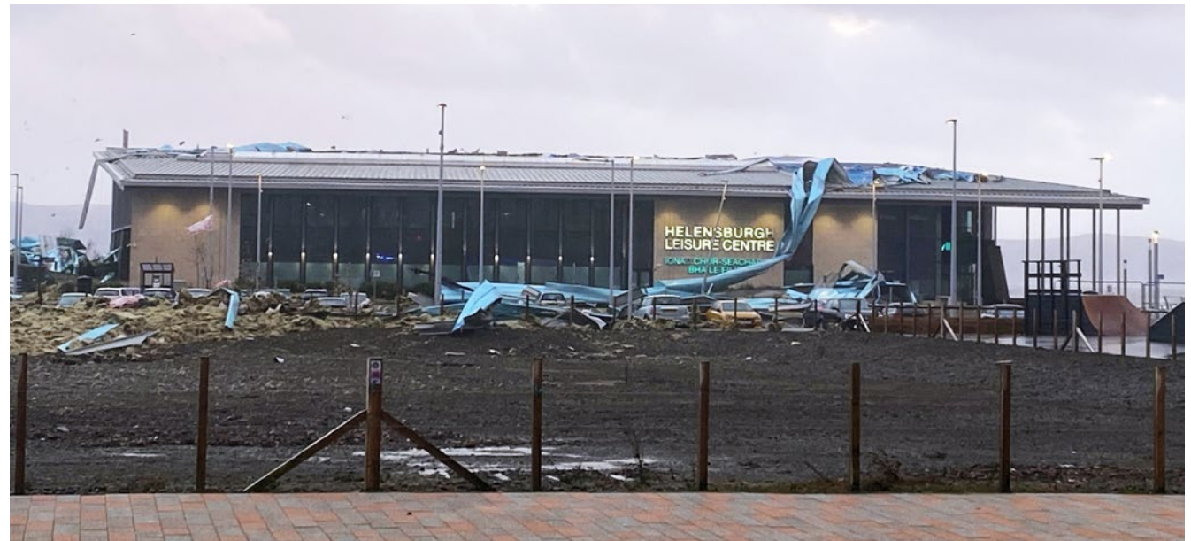
Helensburgh Leisure Centre after Storm Éowyn
