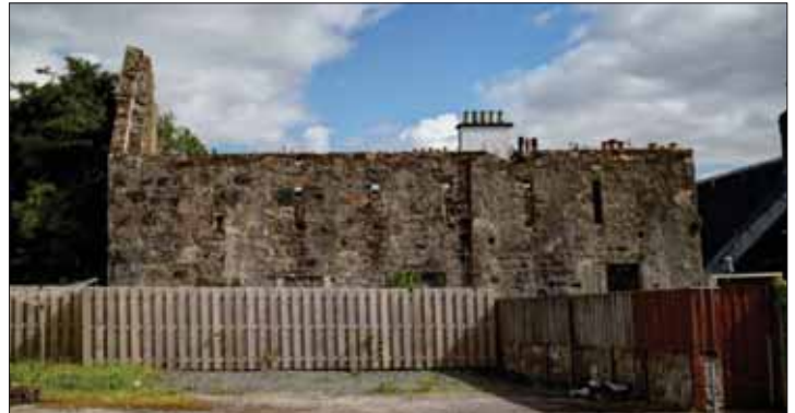
Barn Brae—currently on the Buildings at Risk Register
