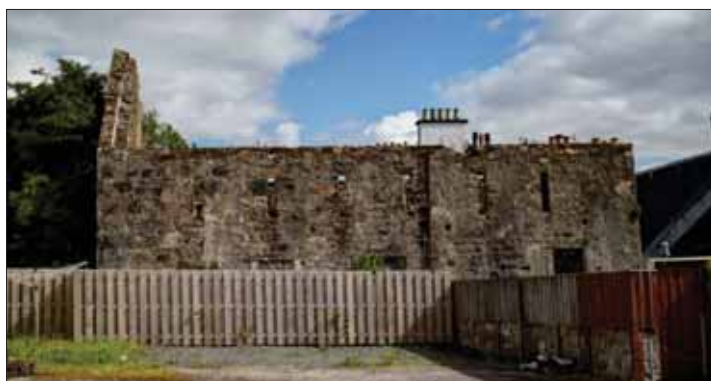
Barn Brae—currently on the Buildings at Risk Register is a threat to the character of the area.
