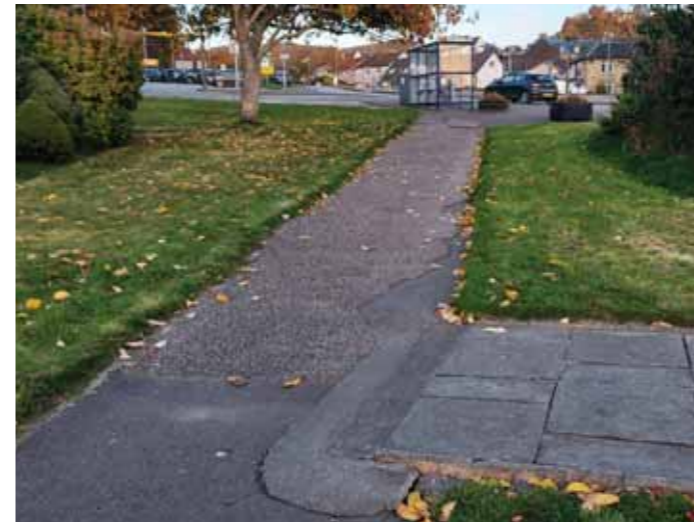
The footway surface is uneven with poor quality paving
