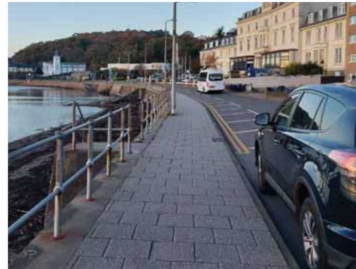
Pedestrian route leading north from Corran Esplanade. The footway surface is slightly uneven
