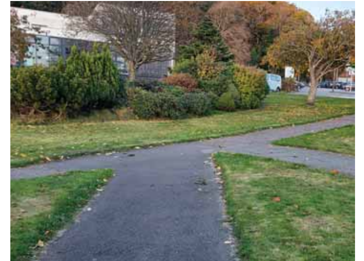
Pedestrian route looking north to Corran Halls with multiple jointed routes in same width
