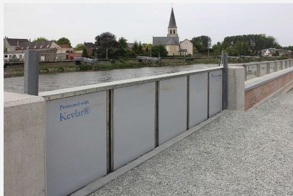
Flood Gate & Transparent Panels
