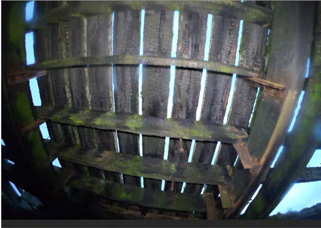
FIGURE 14: Helensburgh Pier – Burnt beams, rafters and floor boards (“C” in Figure 13)
