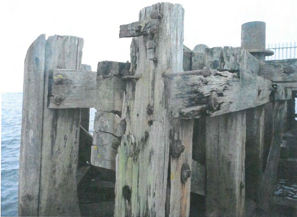
Photograph 1 Rounded post (1-2) as a result of sapwood erosion/decay.
