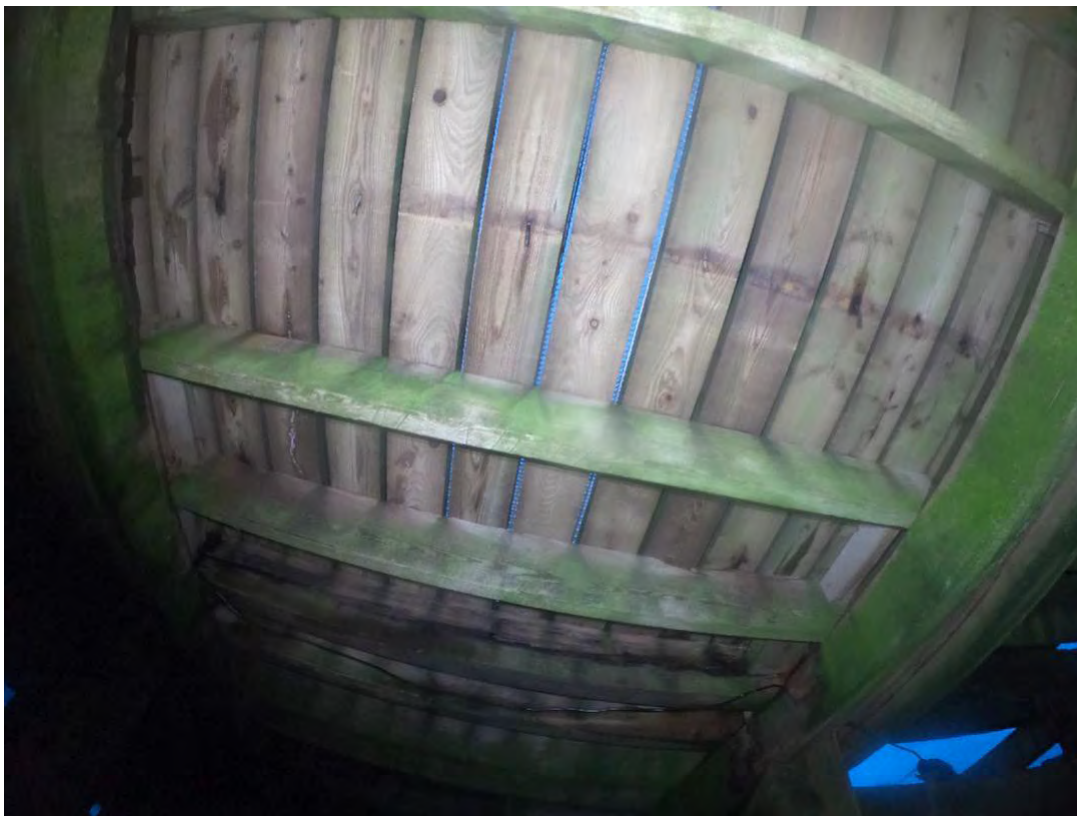
FIGURE 12: Helensburgh Pier – Missing rafter (“B” in Figure 10)
