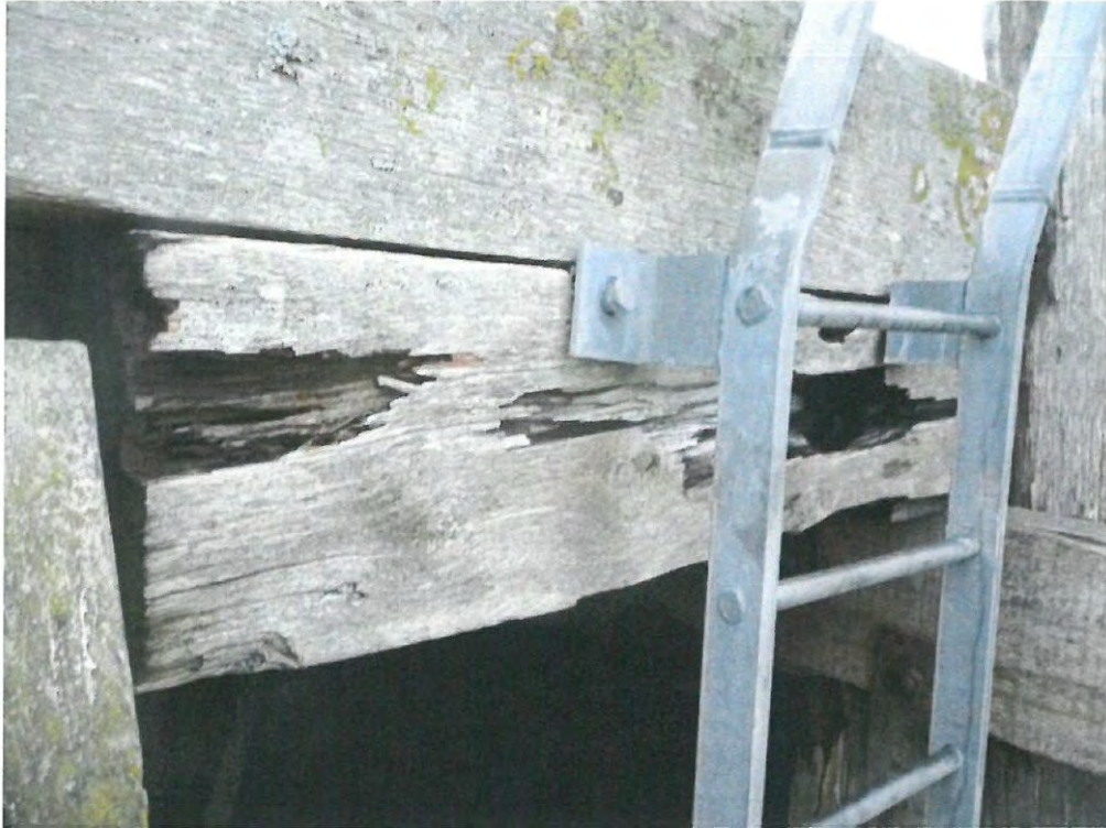
Photograph 9 Significant decay to softwood noggings on the south elevation between piles A-6 and A-8.
