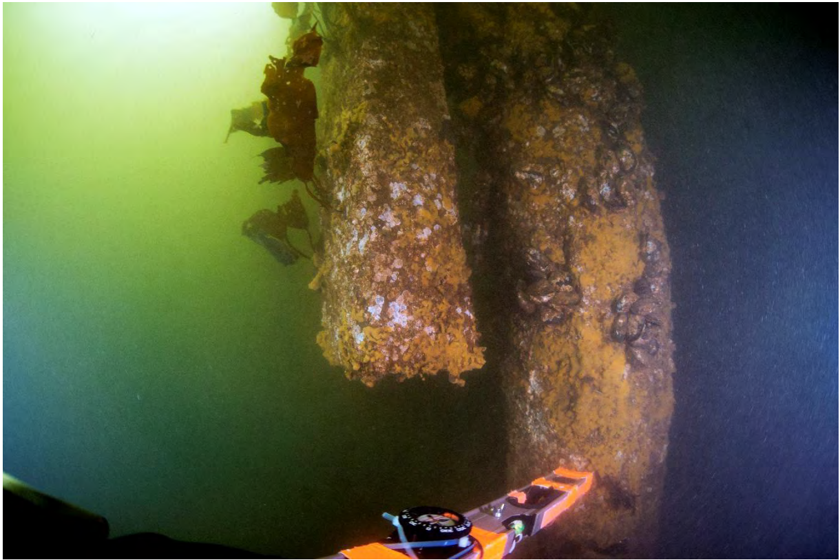
FIGURE 8: Helensburgh Pier – Pile 27 (scale = 58.5 x 6.0 cm)
