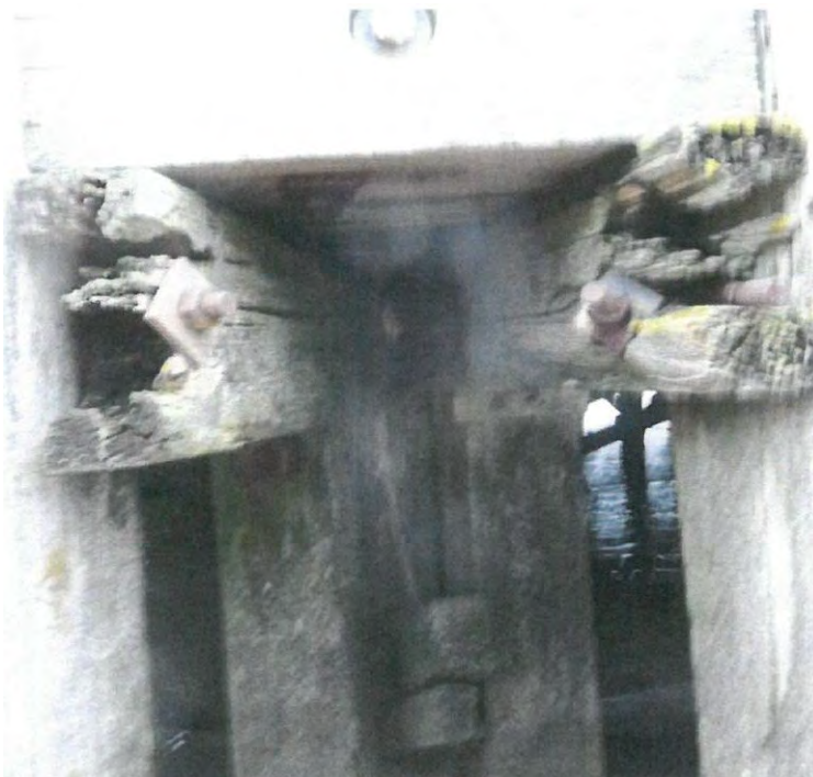
Photograph 10 Significant decay to the south west ends of double deck joists at the south west corner.
