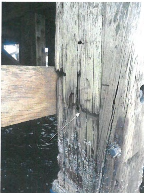
Photograph 2 Significant cross grain fracture to inner pile A-3-b.
