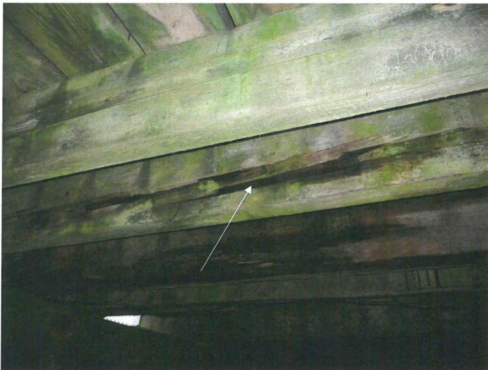
Photograph 15 Example of a softwood deck joist significantly decayed.
