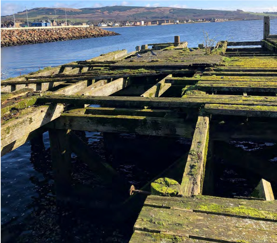
Figure 1.1: Damaged section of timber pier at Helensburgh
