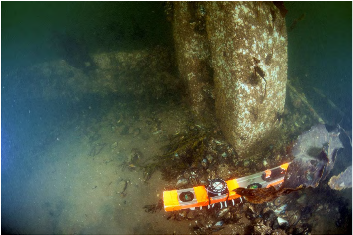
FIGURE 4: Helensburgh Pier – Pile 06 (scale = 58.5 x 6.0 cm)
