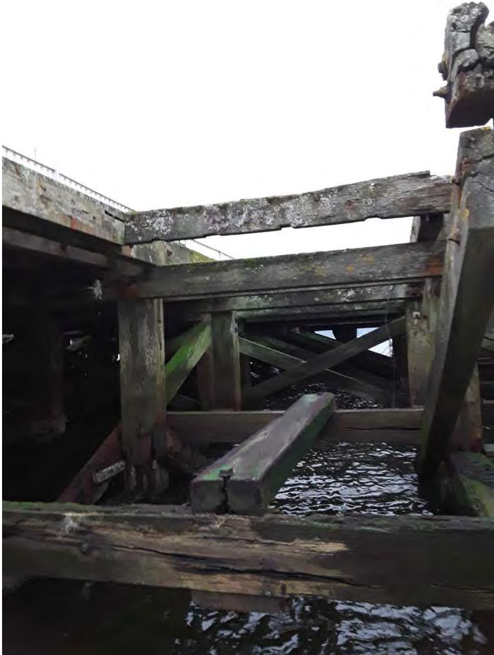
Fire damaged area missing deck planks
