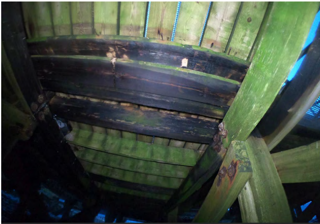
FIGURE 15: Helensburgh Pier – Burnt rafters (“D” in Figure 13)
