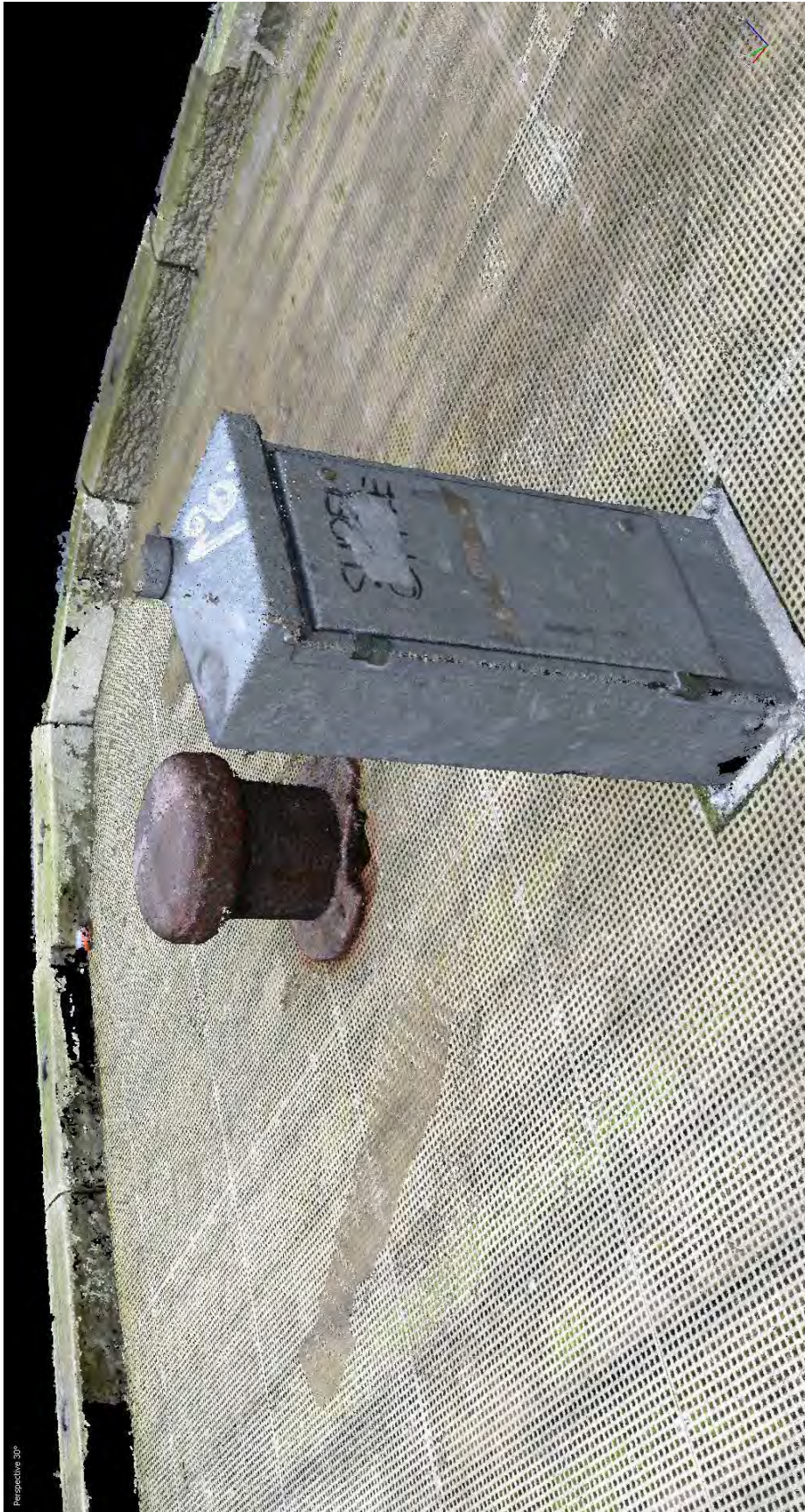
FIGURE 24: Helensburgh Pier – Screen grab of deck bollard damage
