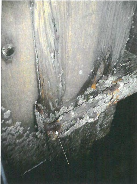
Photograph 5 broken steel strap around pile D-13.
