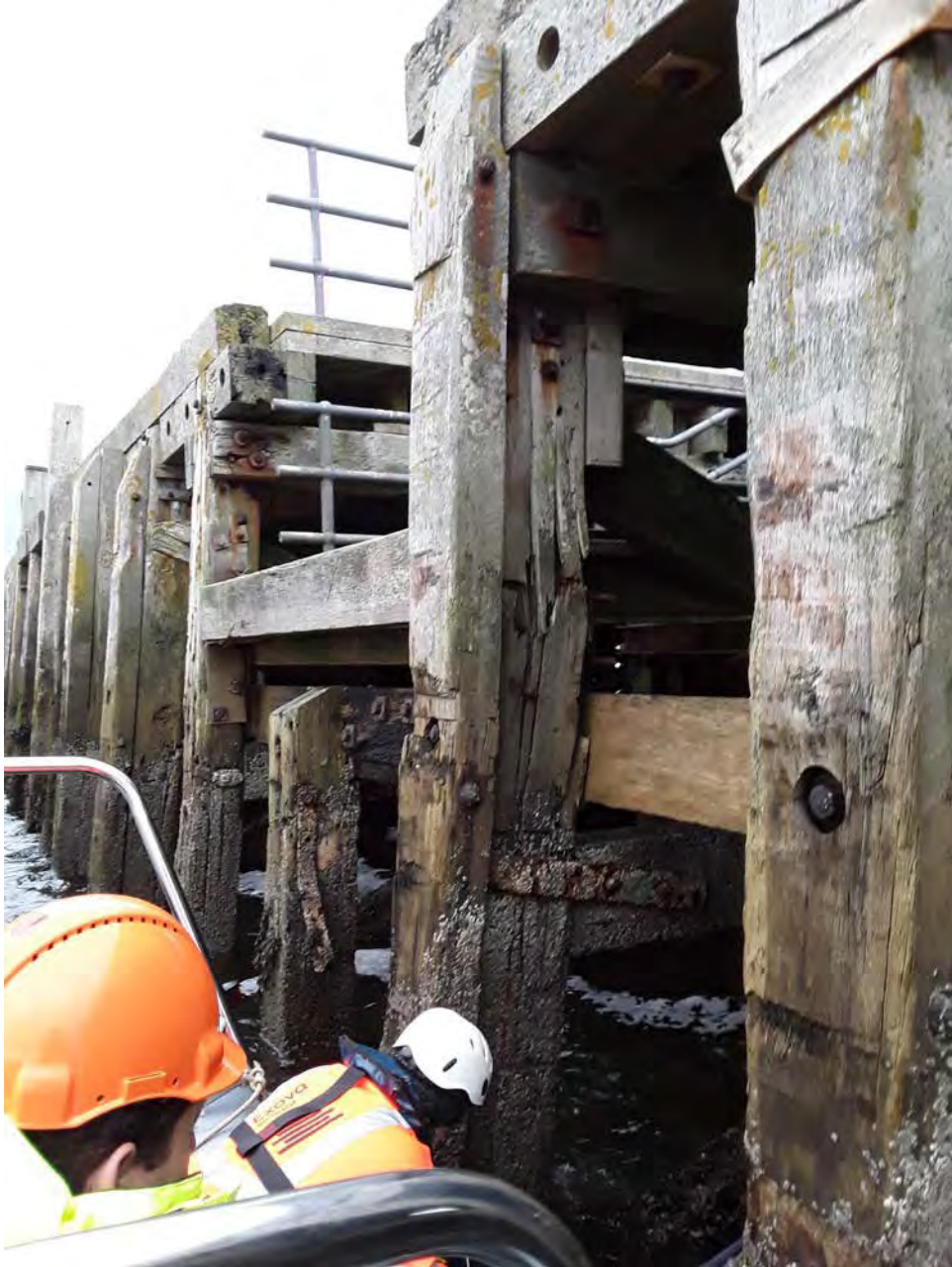
Splitting across the grain of timber fender from impact damaged, adjacent to stairs.
