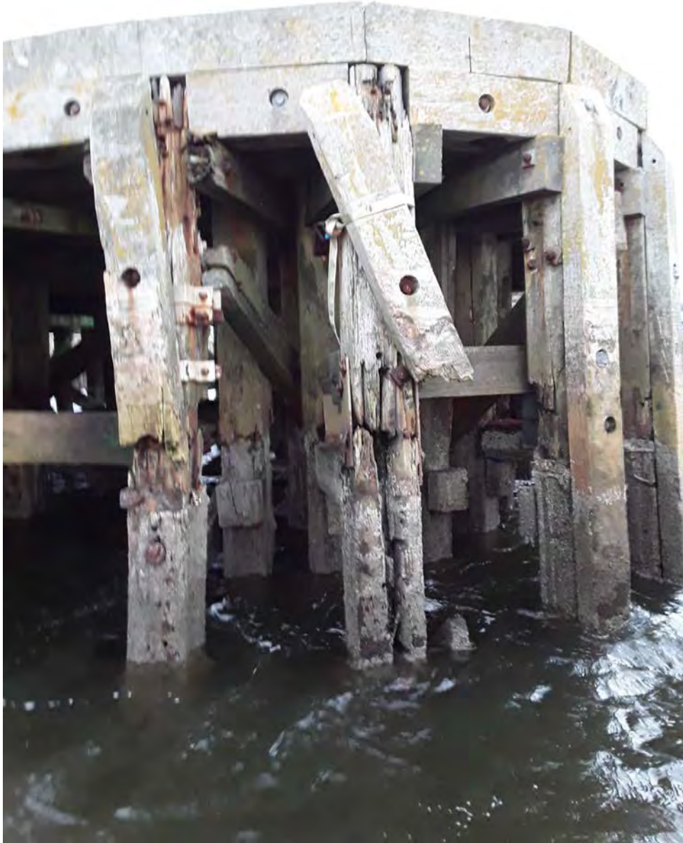
South east corner pile and fender impact damage and previous repairs
