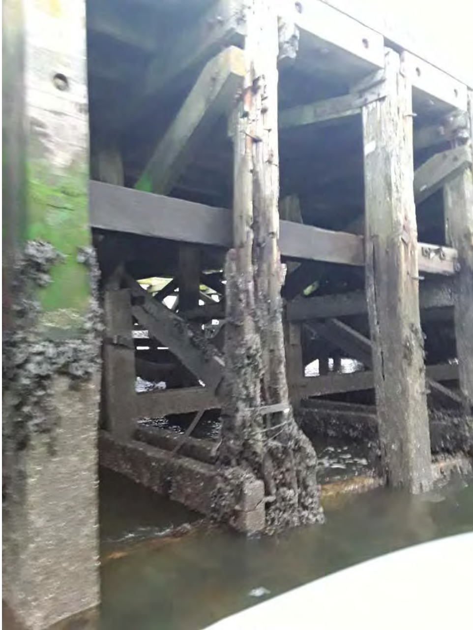
Pile section loss at west end of southern berthing face
