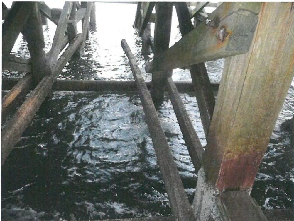
Photograph 8 Horizontal beam C-6 to E-6 disconnected.
