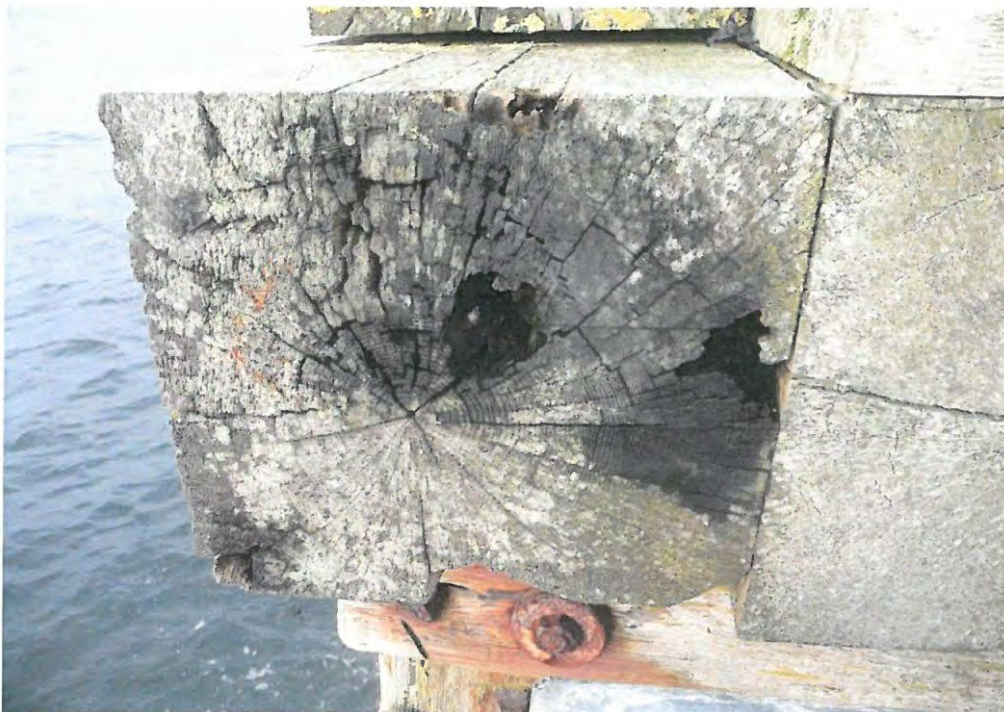
Photograph 12 Fungal decay seen at end grain of a softwood nogging on the south elevation.
