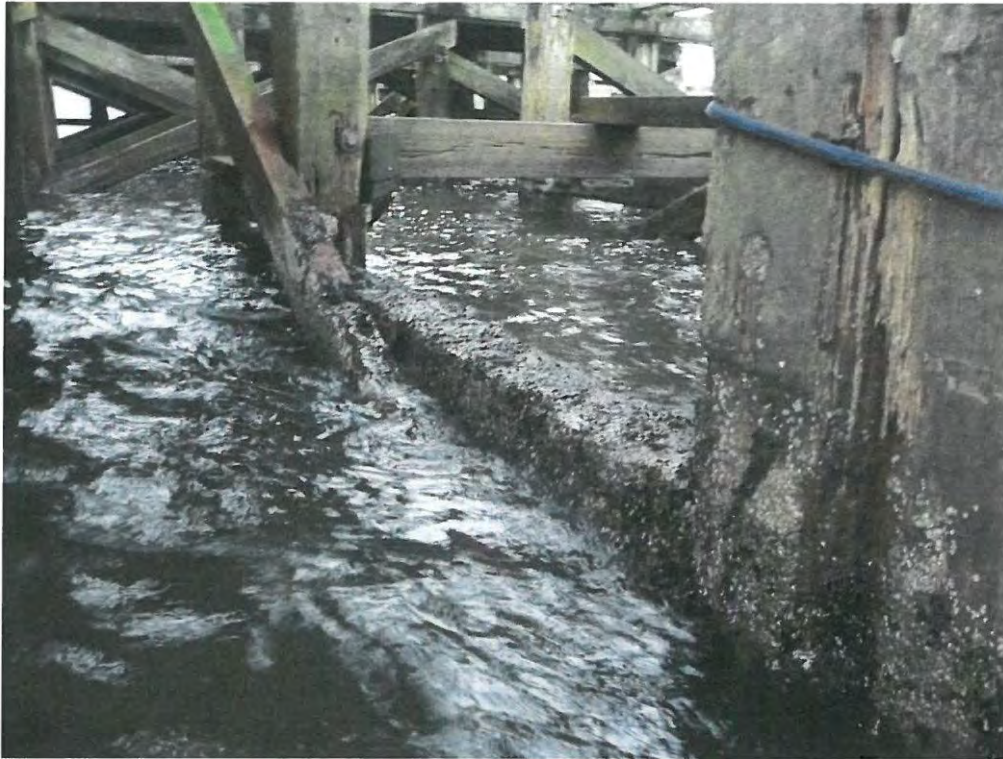
Photograph 7 Mid horizontal E-1 to E-2 dropped from original position.
