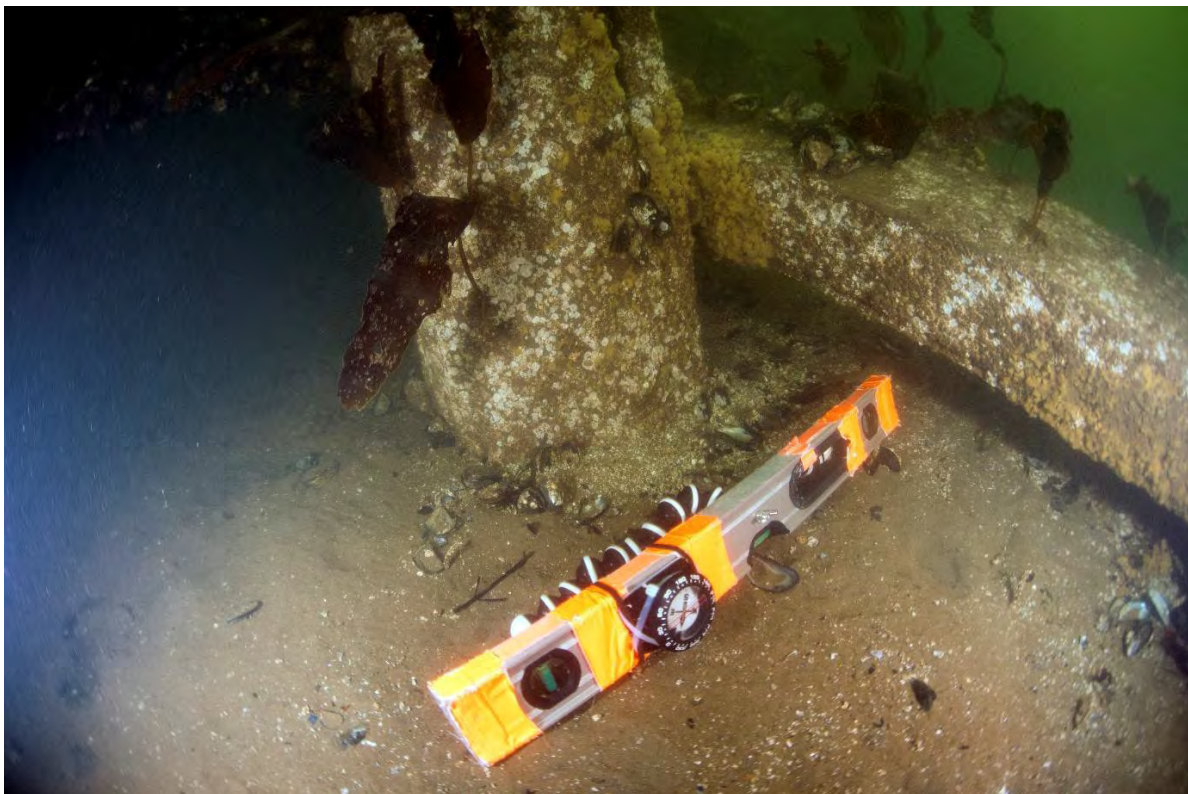
FIGURE 3: Helensburgh Pier – Pile 05 (scale = 58.5 x 6.0 cm)
