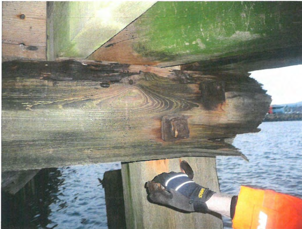
Photograph 13 Example of a softwood double deck joist significantly decayed.
