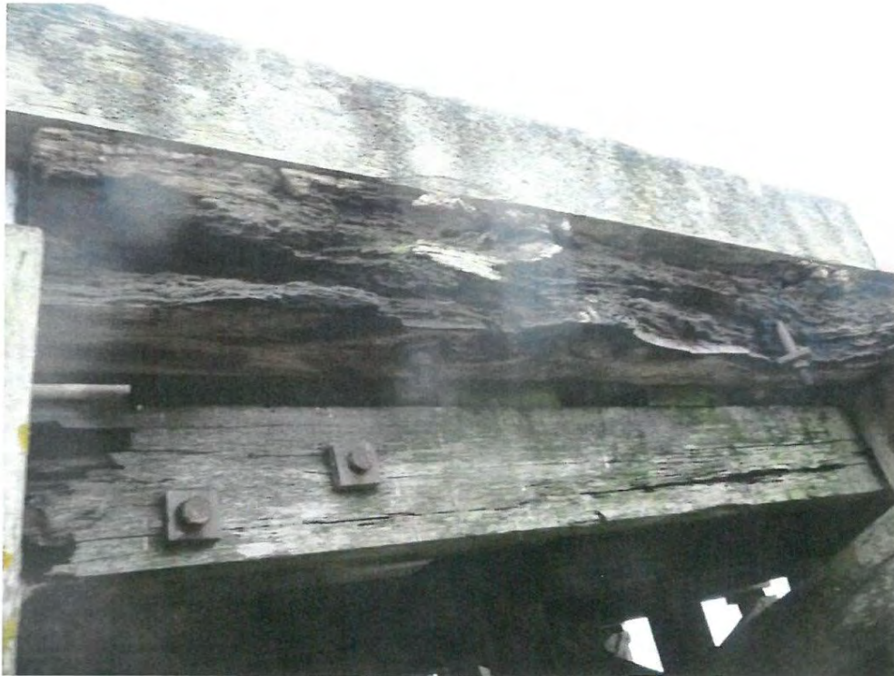
Photograph 11 Significant decay to nogging on west elevation and horizontal member below.
