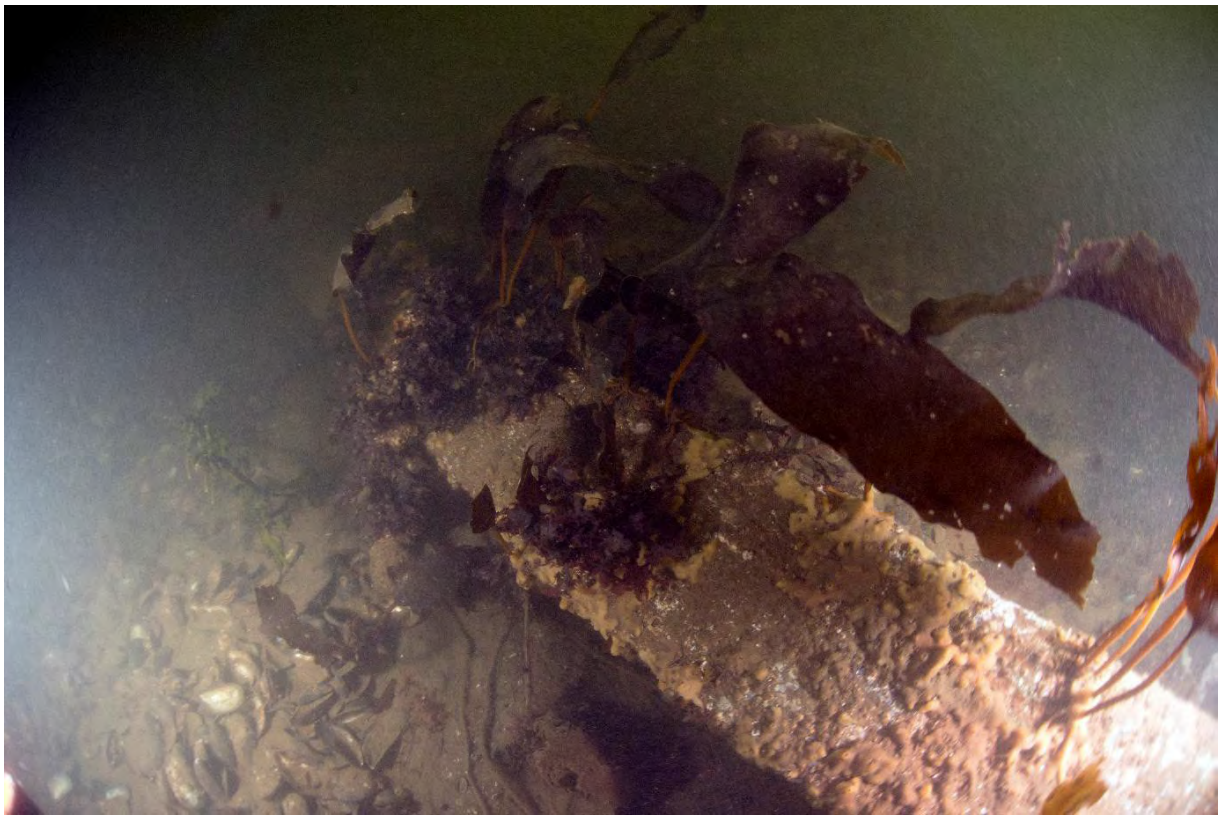
FIGURE 6: Helensburgh Pier – Between piles 37 and 38 (37-b.jpg)
