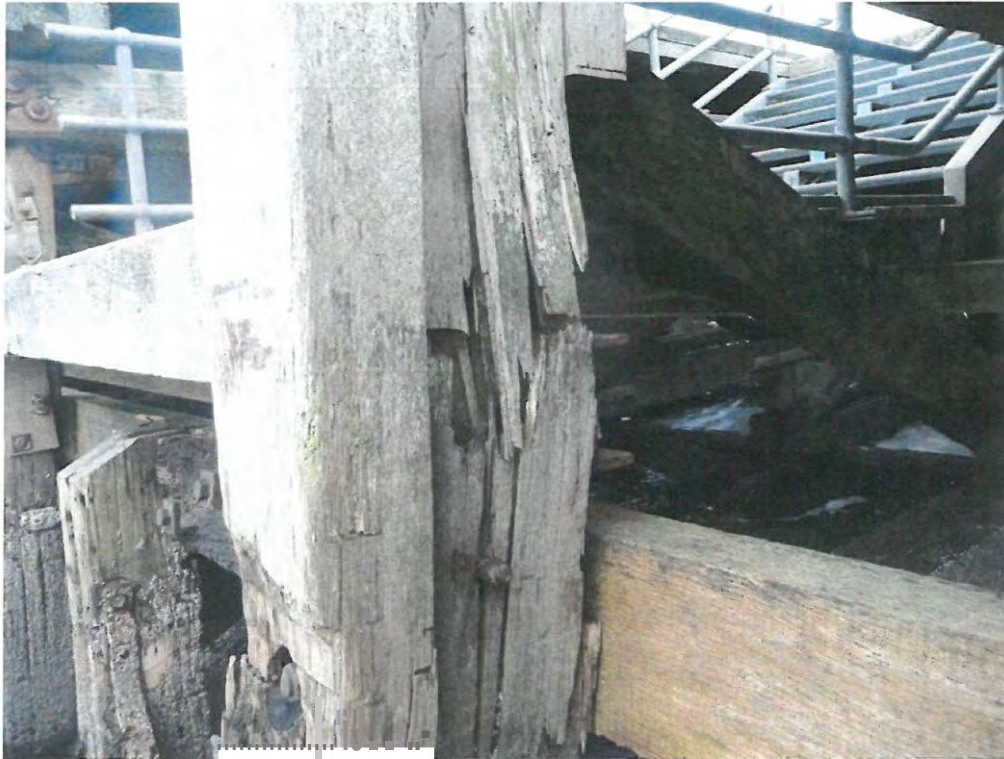
Photograph 3 Significant cross grain fracture to inner pile A-4-a.
