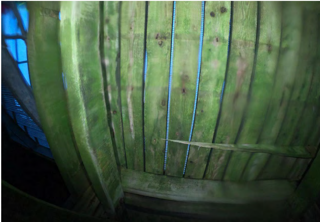
FIGURE 11: Helensburgh Pier – Missing and broken rafters (“A” in Figure 10)
