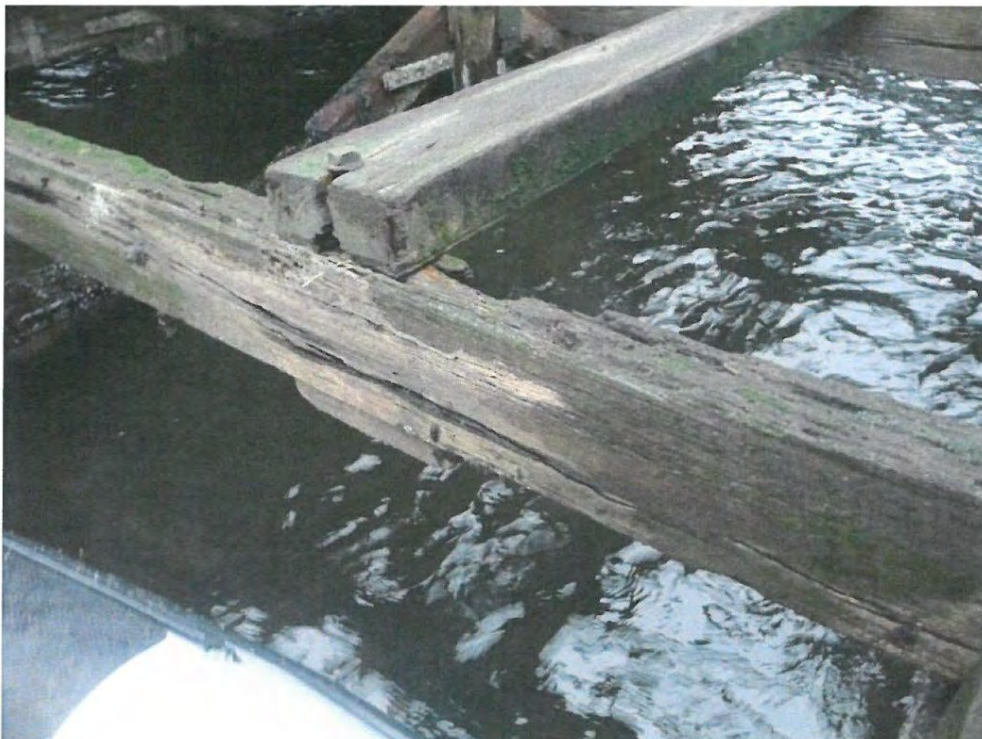
Photograph 6 Example of significant decay and erosion to mid horizontals E-1 to F-1, E-2 to F-2 and F-1 to G-1.
