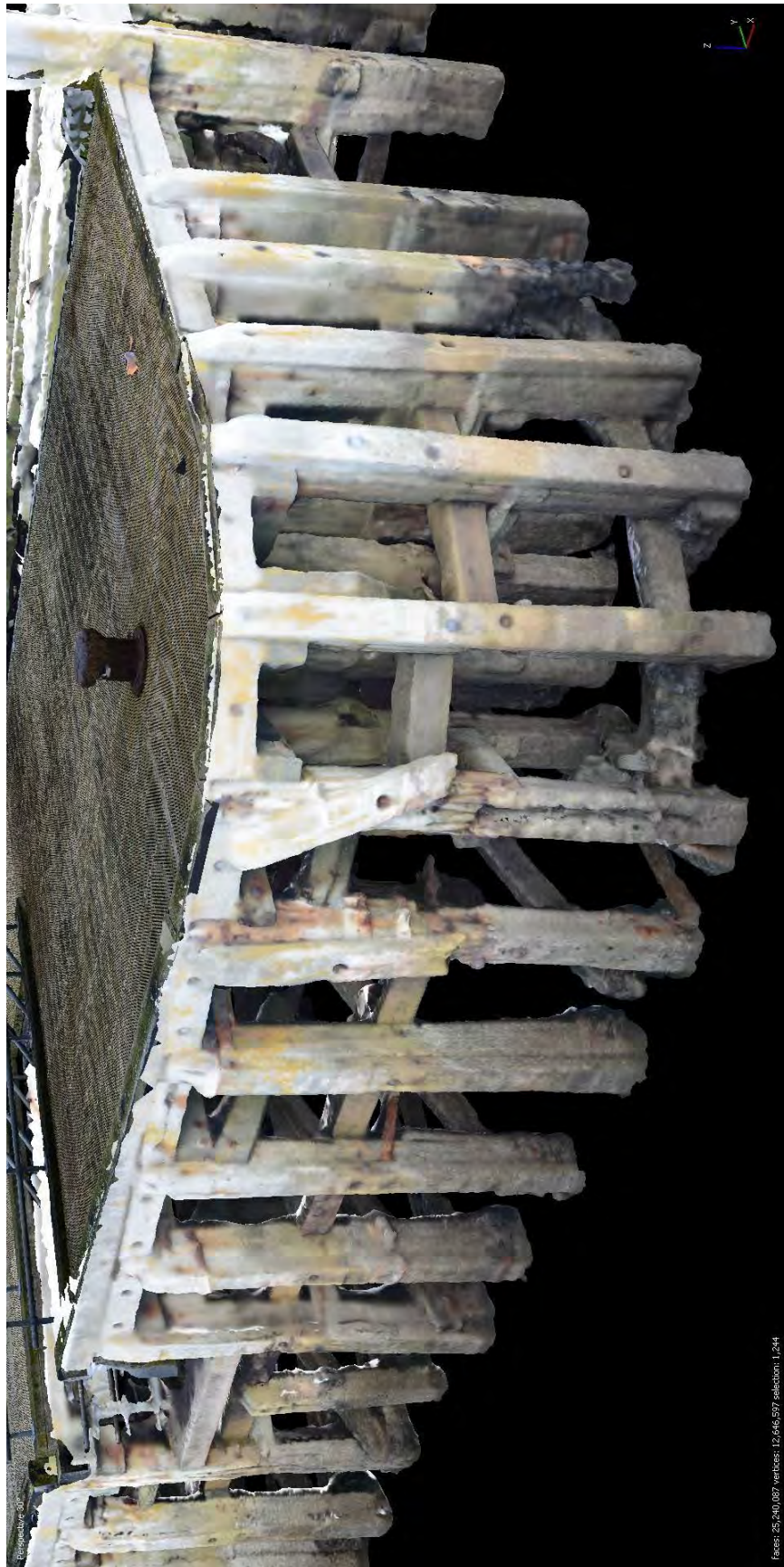
FIGURE 23: Helensburgh Pier – Screen grab of exterior piling damage
