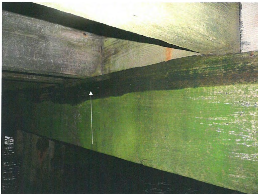
Photograph 16 Example of a softwood double deck joist significantly decayed.
