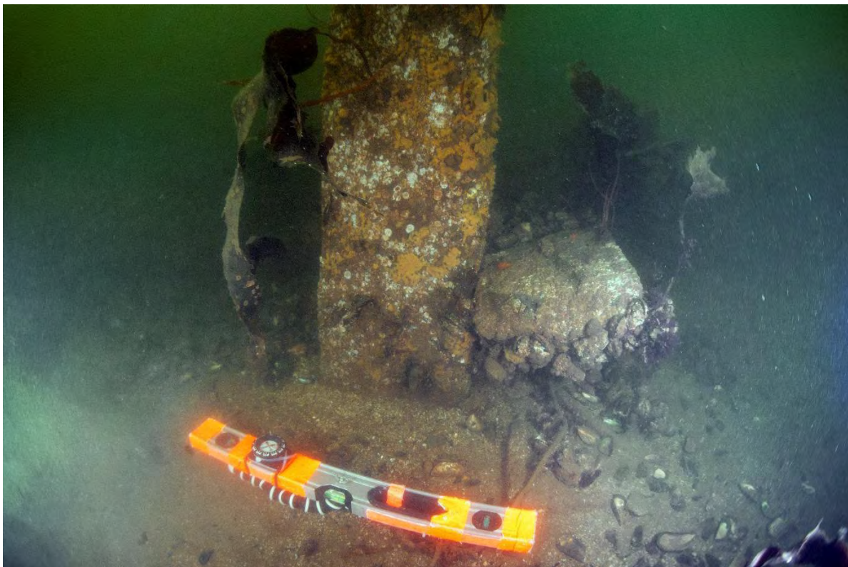
FIGURE 7: Helensburgh Pier – Pile 41 (scale = 58.5 x 6.0 cm)
