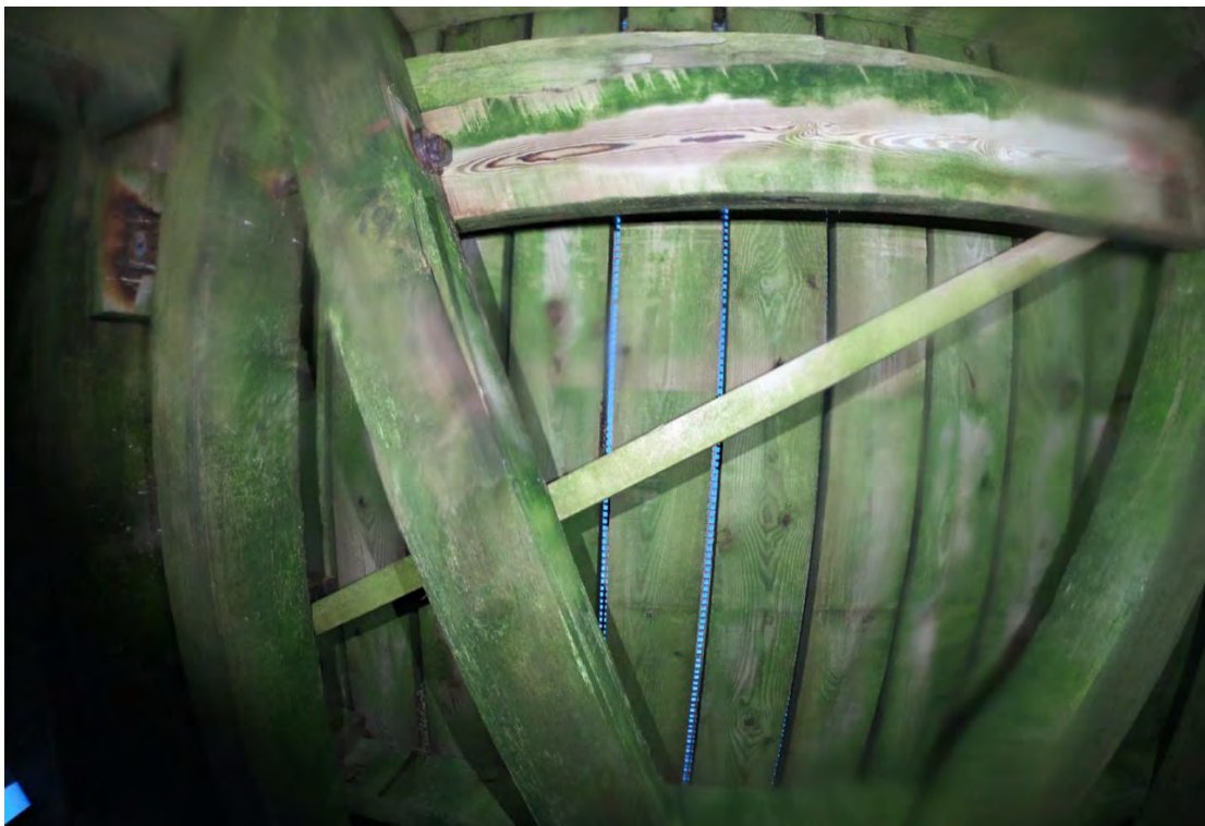
FIGURE 18: Helensburgh Pier – Misaligned rafters (“F” in Figure 16)
