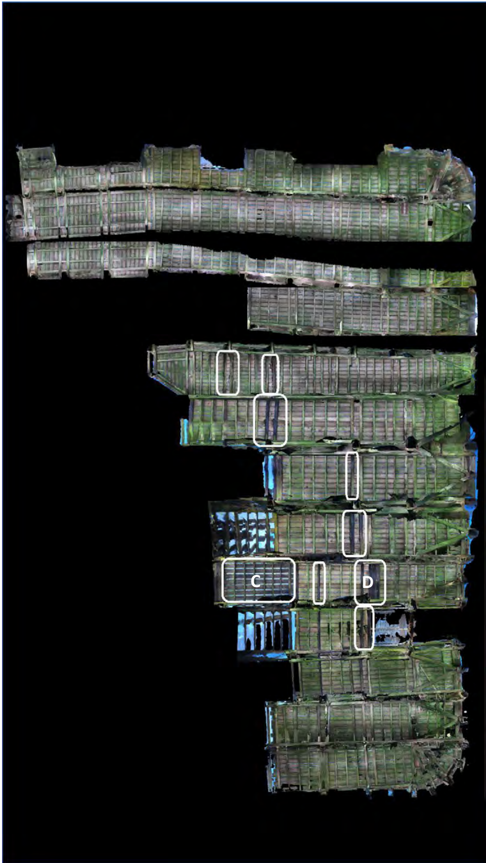
FIGURE 13: Helensburgh Pier – Composite image of the underside of the pier showing areas with presumed fire damage (in white)
