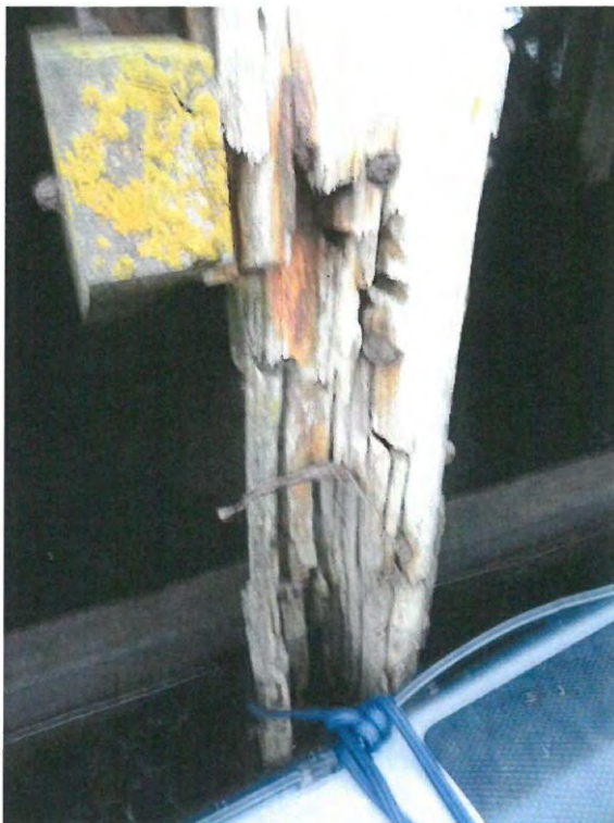
Photograph 4 Significant loss of cross section due to impact damage and erosion to pile A-11-a.
