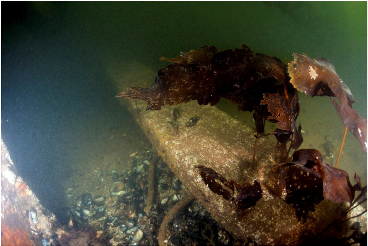
FIGURE 2: Helensburgh Pier – Between piles 04 and 05 (04-b.jpg)
