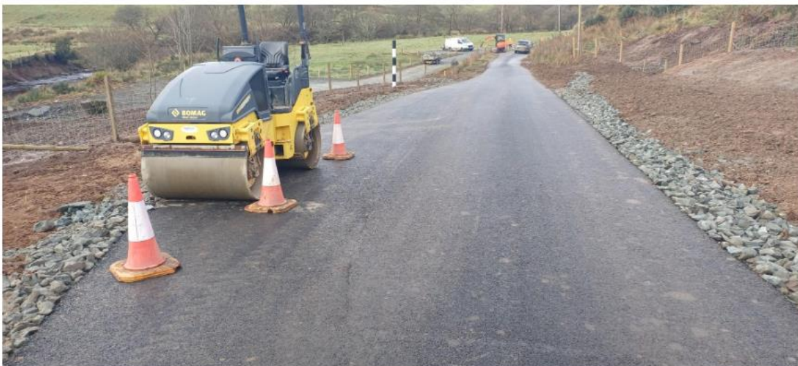
New lowered road alignment and improved drainage with slope strengthening and additional passing place - completed in November 2024.
