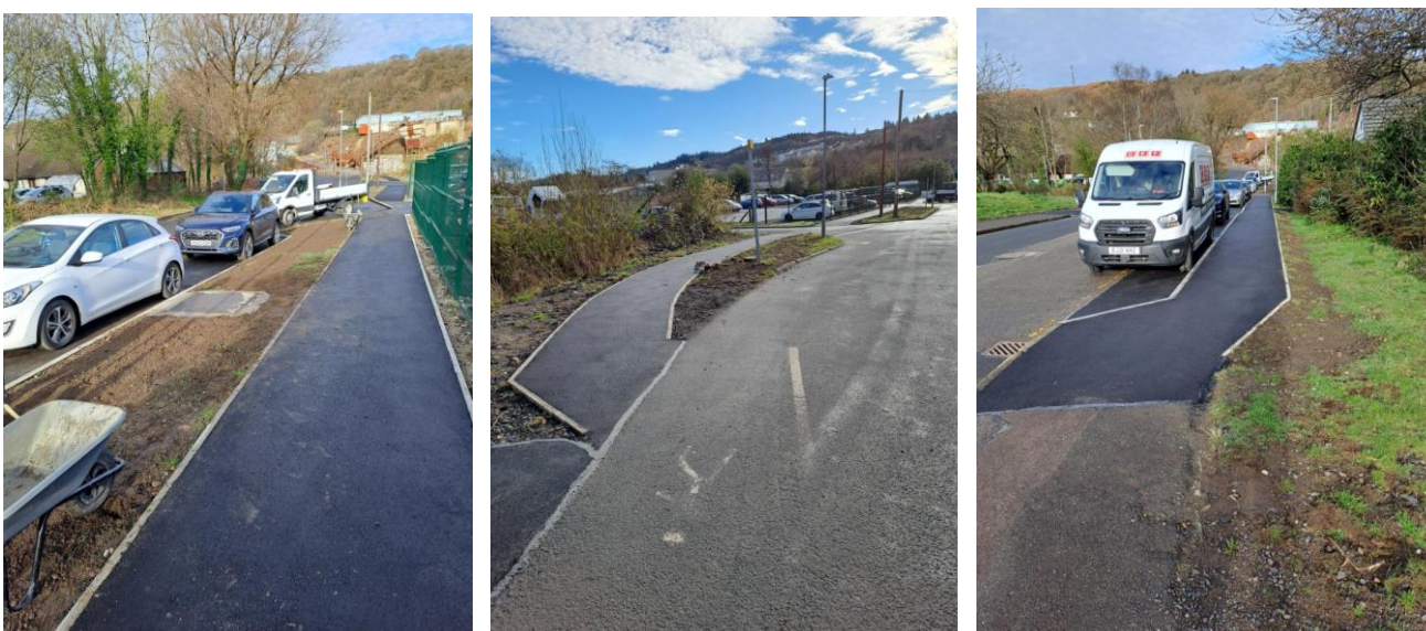
Millpark Road – Oban – Linking footpaths and on-street parking improvements T.S. Safety fund.
