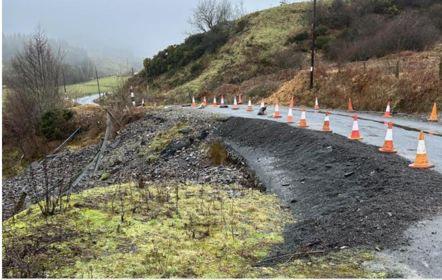
Existing unstable slope, subject to frequent movement.
