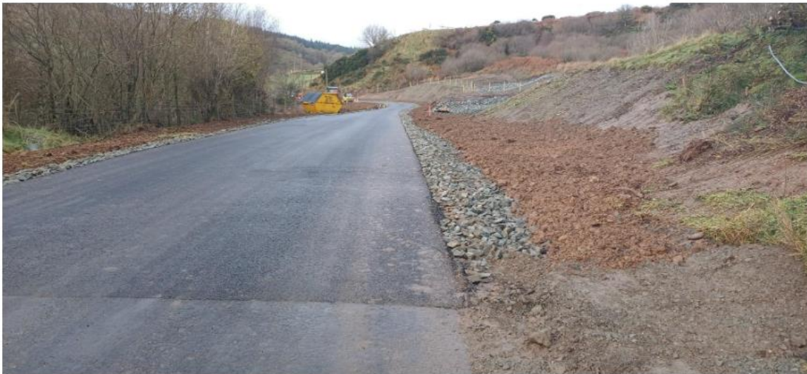
Looking south, showing extent of road realignment and slope reprofiling and strengthening. Work complete in November 2024.
