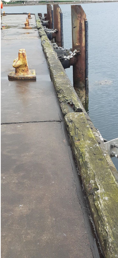
Image B3. Campbeltown, New Quay wooden edge beams
