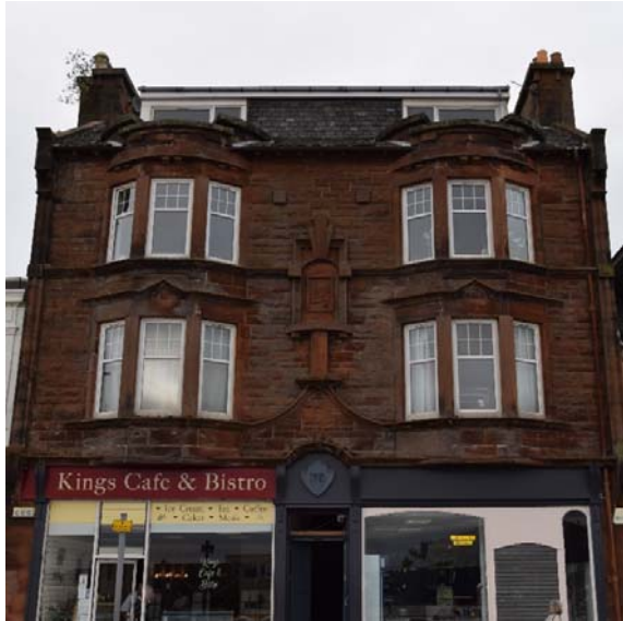
17-19 West Clyde Street (Category B listed). Typical building failures include vegetation growth, failure of roof details and repairs. Significant stone repair and structural intervention is required with movement evident to canted window bays.
