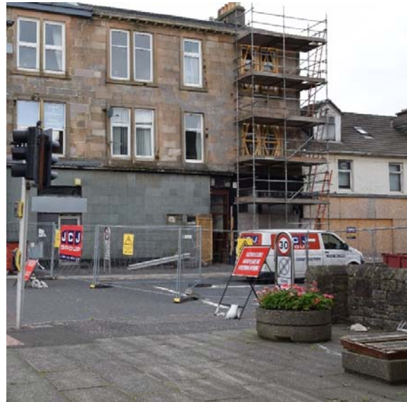
5-7 East Clyde Street. A dangerous building notice has been issued on the building. Without a comprehensive fabric repair programme the building is in risk of full demolition in the future.
