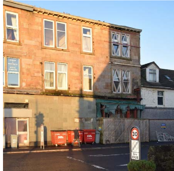
5-7 East Clyde Street. Building subject to emergency notice from Argyll and Bute Council. Works include doughtakings to gable, propping of internal pen check stair and propping of shop lintel.
