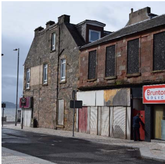
The vacant ground floor shops to 1-5 Colquhoun Street has a negative impact on the perceived quality of the area. The vacancy to upper levels indicates to visitors that this isn't a High Street issue of not being able to let the unit but a much wider condition issue.
