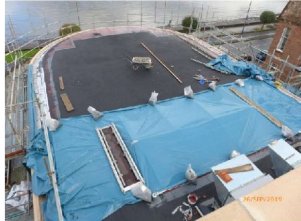
Looking East: General View of the north roof over the Exhibition/Function Suite.
