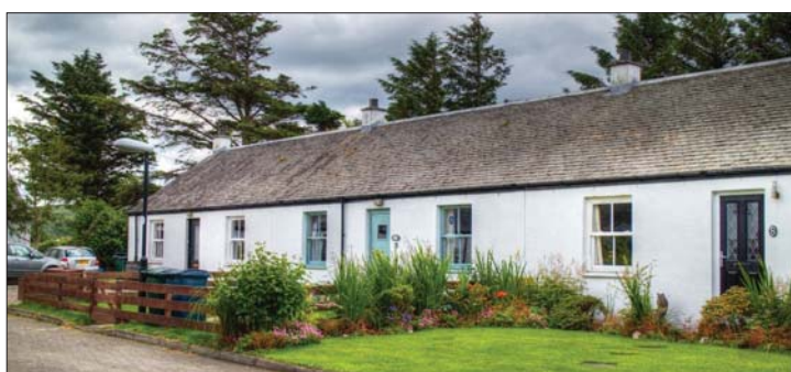
New, inappropriately small, chimneys
