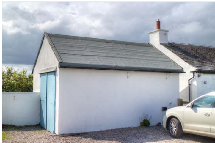
Inappropriate felt roof
