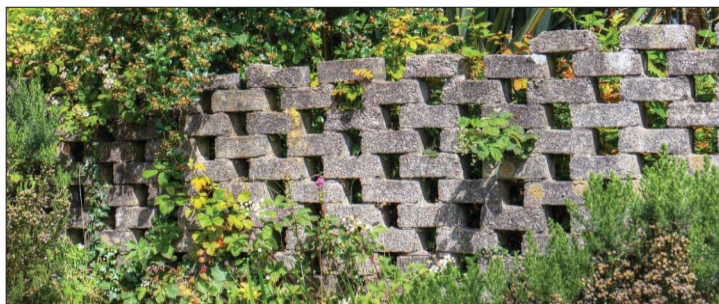
Inappropriate concrete wall
