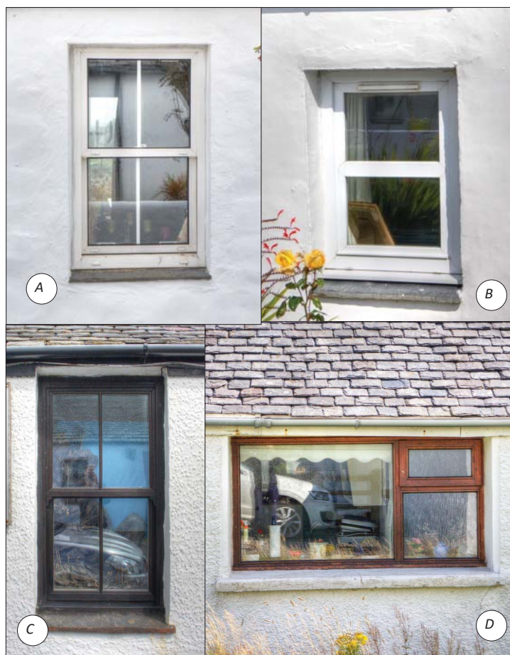
Inappropriate windows: A—uPVC with stuck on astragals B—uPVC with visible trickle vent C—uPVC with horns D—horizontal orientation
