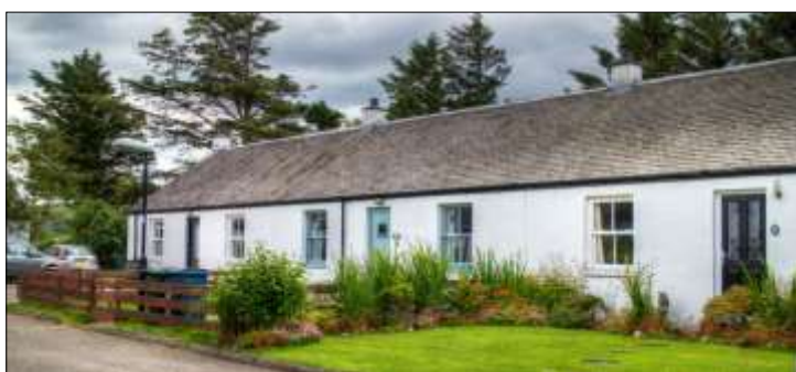
New, inappropriately small, chimneys
